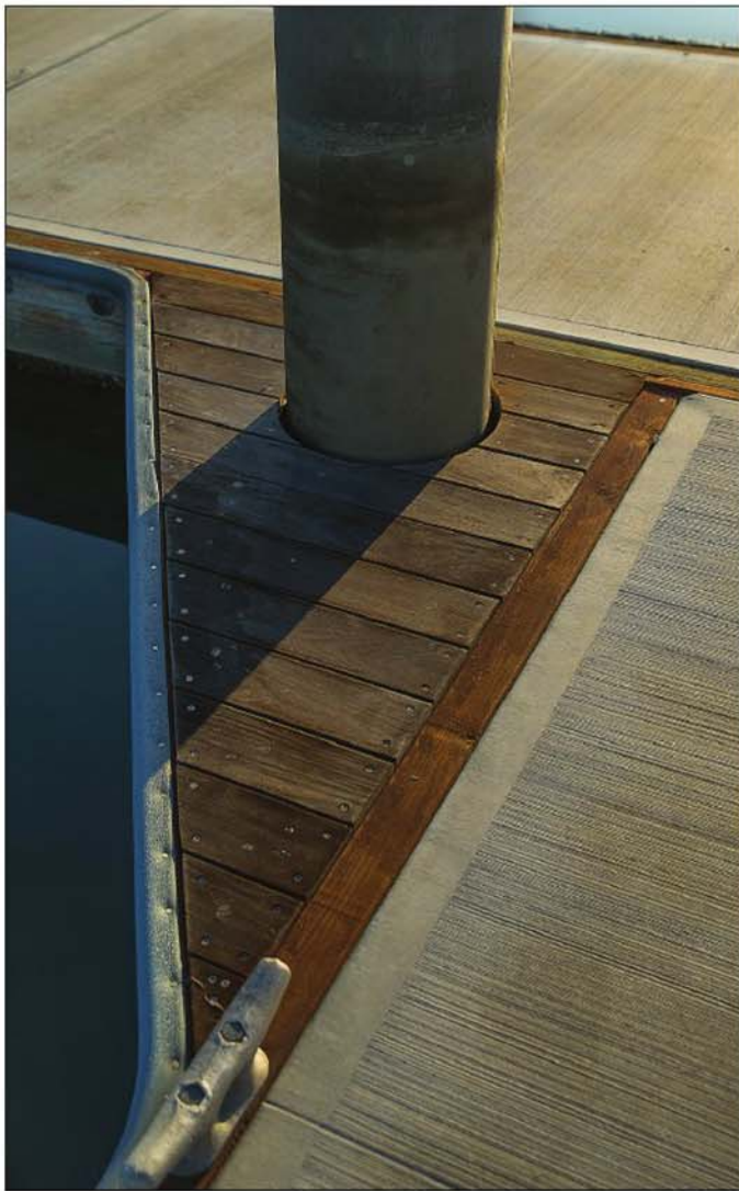
Single-piece finger piers with rounded ends and warm wood trim make up the clean lines of the floating concrete docks. The rounded piling are internally mounted, and an HDPE ring, mounted under the dock, acts as a bearing and scrapes the pile clean of shell life.
